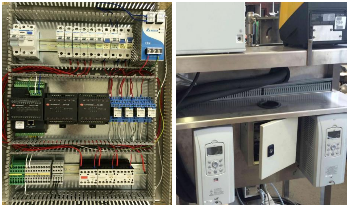
Figure 15: Electrical cabinet and VSD's (Smith, 2014)
