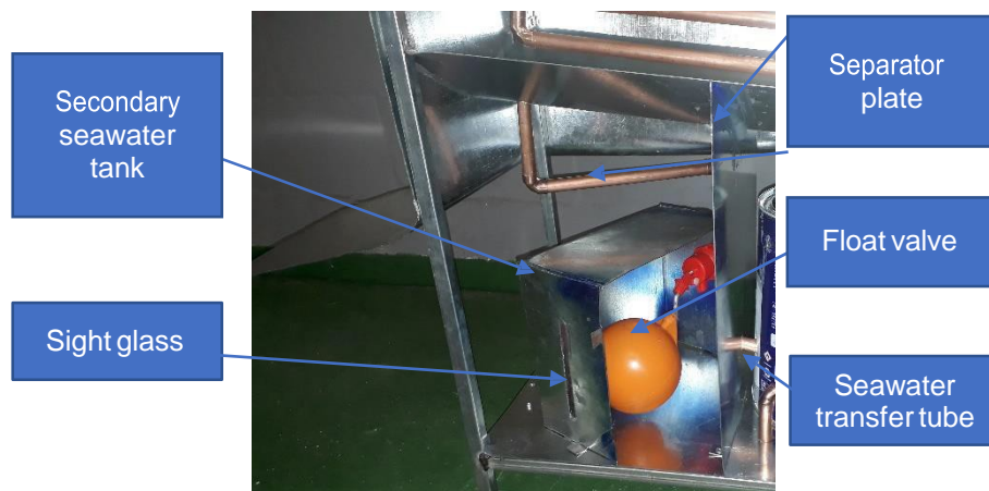
Figure 3.25: Seawater tank and float valve
