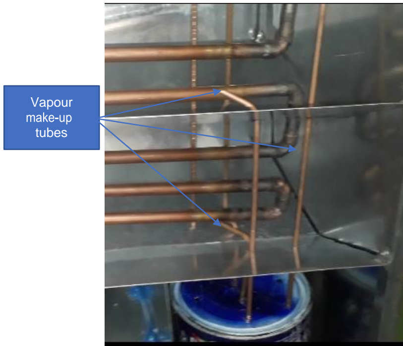
Figure 3.23: Vapour make-up tubes
