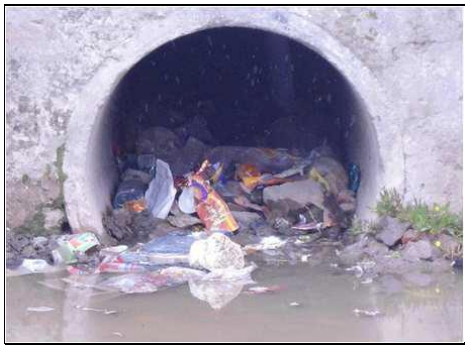
Blockages to the bulk system due to illegal dumping/ littering causing localised flooding
