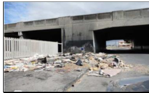
Illegal dumping occurring in Netreg road under the bridge
