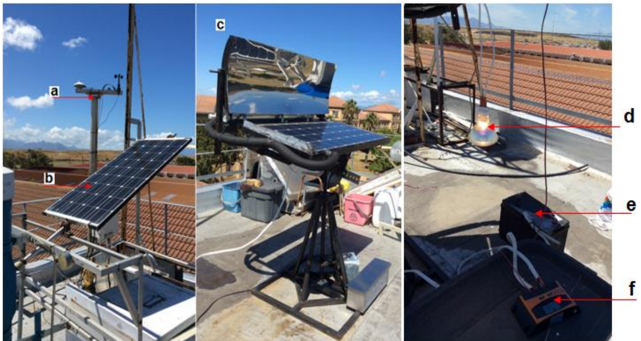
Figure 4-1: Experimental set-up prototype a) Weather station; b) Semi-fixed PV; c) CSPVT; d) DC bulb e) DC battery; f) Charge Controller
