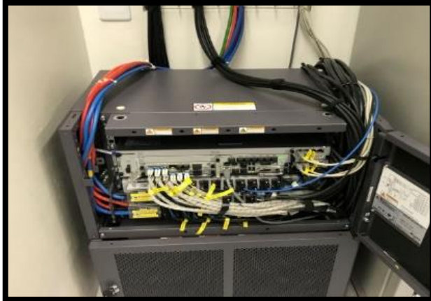
Figure 1.2: eNodeB baseband unit sample site Huawei
