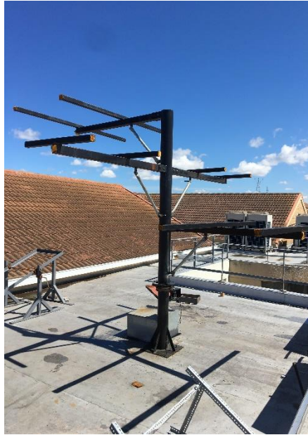
Figure 4.1: Pillar solar tracking system
