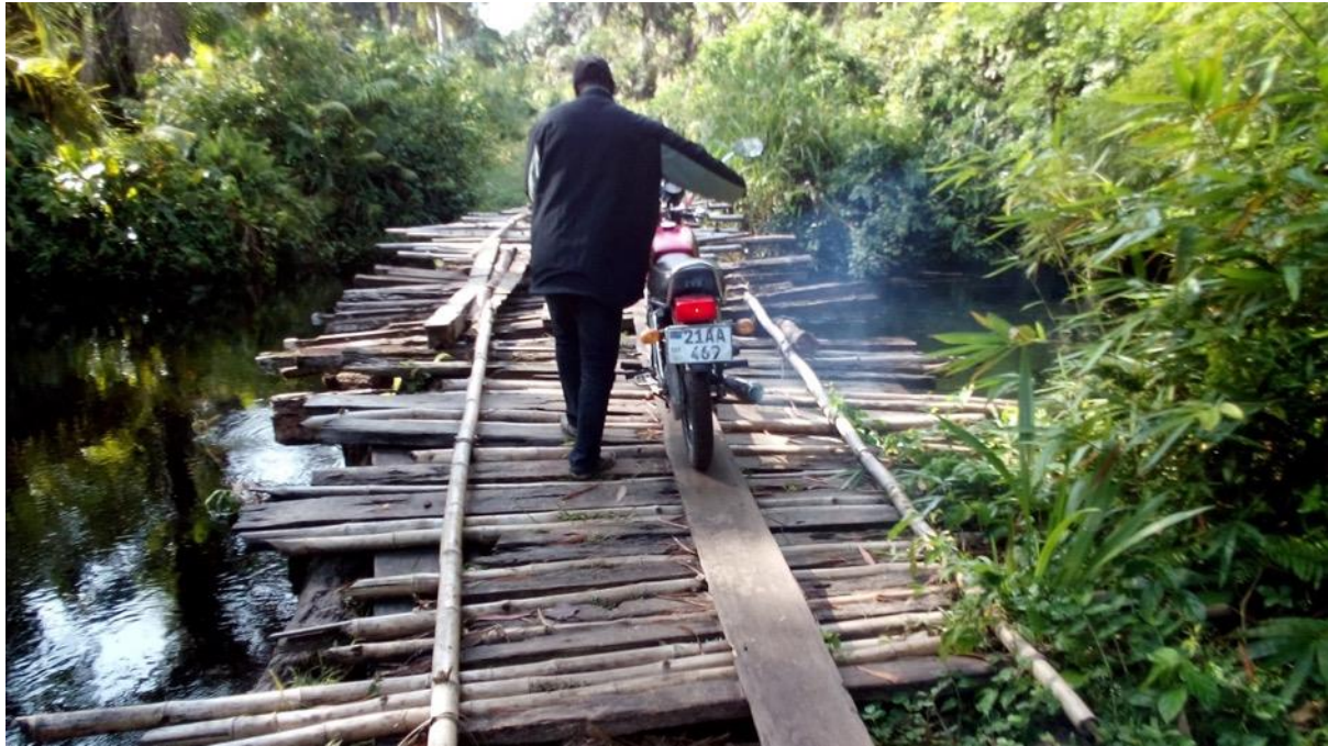
Figure 4.24: One of the many dangerous bridges (Photograph: Lodi Paul Inga, 2016)
