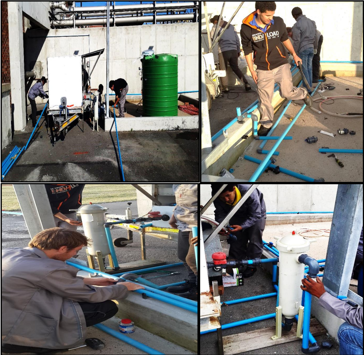
Photograph 3. 2: RO Pilot-plant installation next to the MBR plant with RO plant piping connection.
