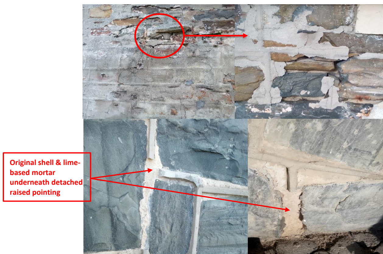
Figure 3.5 Recent failing repairs – Robben Island
