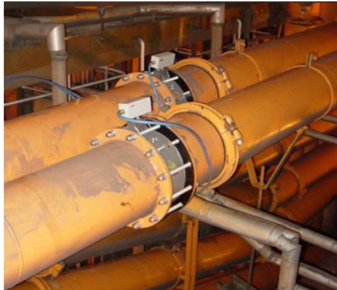
Figure 2.3: PF Flow Meter (ABB, 2018)
