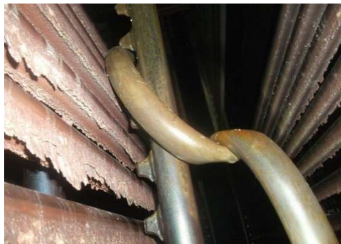
Figure 1.7: Slagging on the super-heater's tubes (Tootla, 2015)
