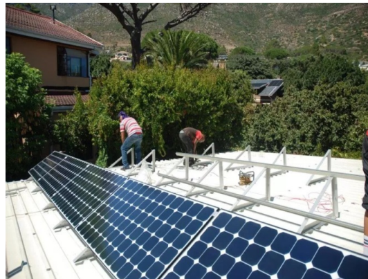
(b) Rooftop PV with structure
