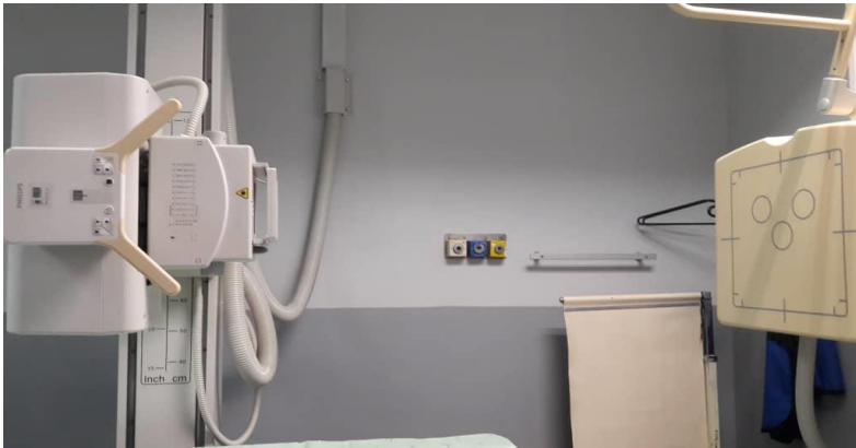
Figure 3.6 Philips Duradiagnost 4 at research site 3
