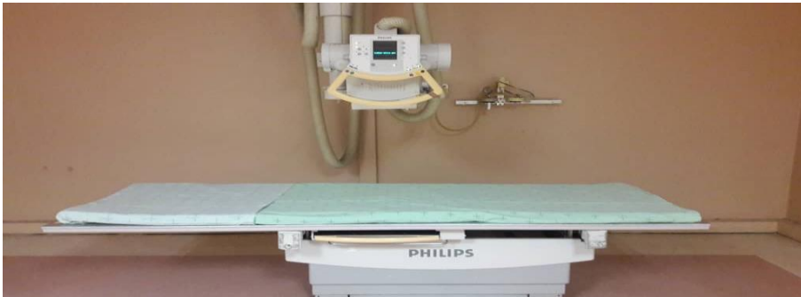
Figure 3.2 Philips Duradiagnost at research site 1
