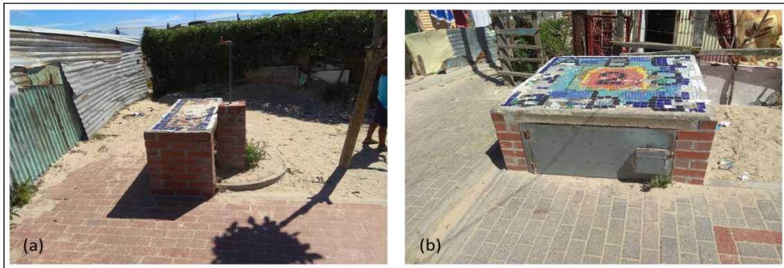
Figure 4:51 : Emthonjeni fitted standpipe and greywater disposal manhole.
