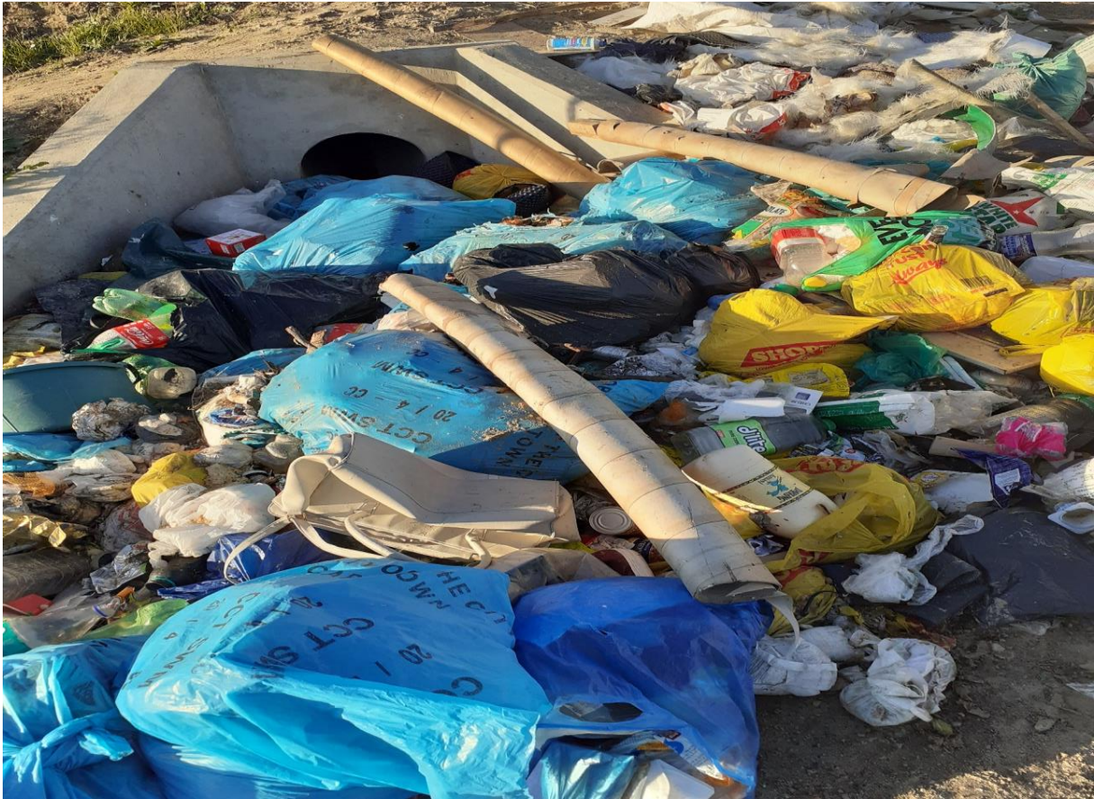
Figure 4.14: Closest drain to the river near Malibongwe Drive bridge
