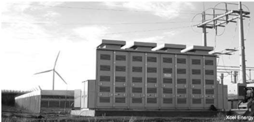
Figure 2-19: 6 MW, 8 h Sodium-sulphur energy storage facility in Tokyo, Japan (Tong, 2010)
