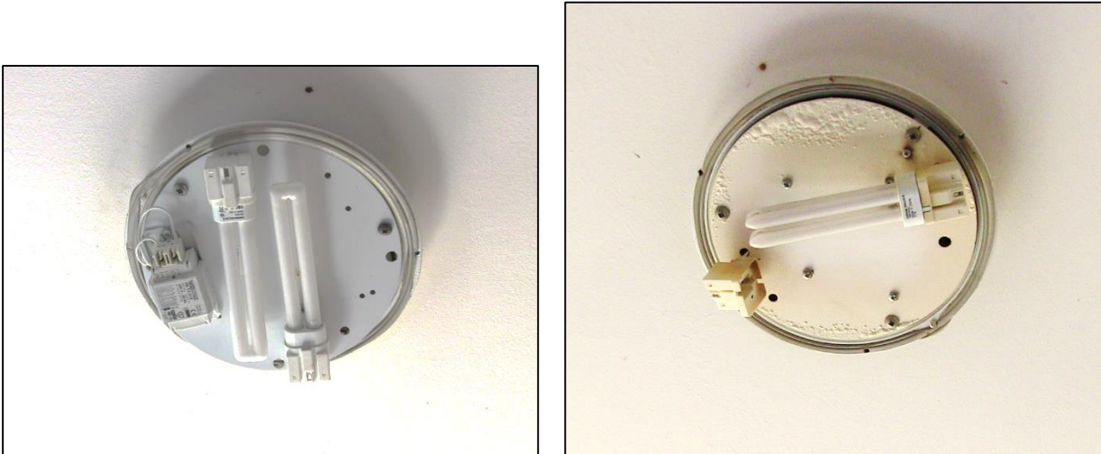
Figure 4.2: Lamp Fittings used in the student rooms (Lokailwe, 2019)
