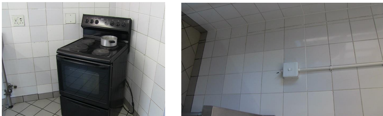
Figure 4.12: Four plate electric stove (left) and the stove is missing (right)
