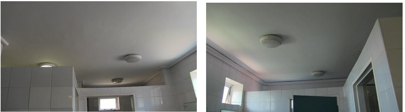
Figure 4.15: Lamp fittings in the restrooms (Left: ON and Right: OFF)
