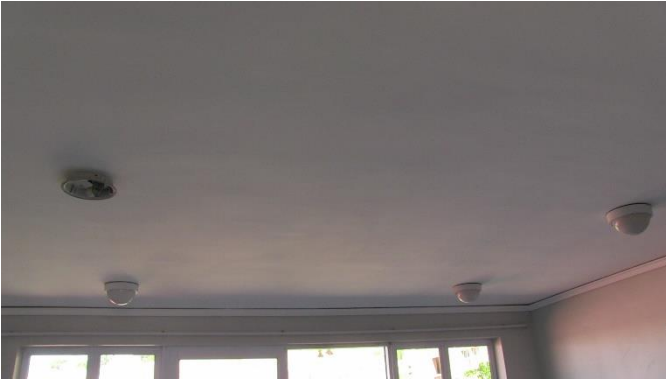
Figure 4.18: Lamp fittings in the recreation area
