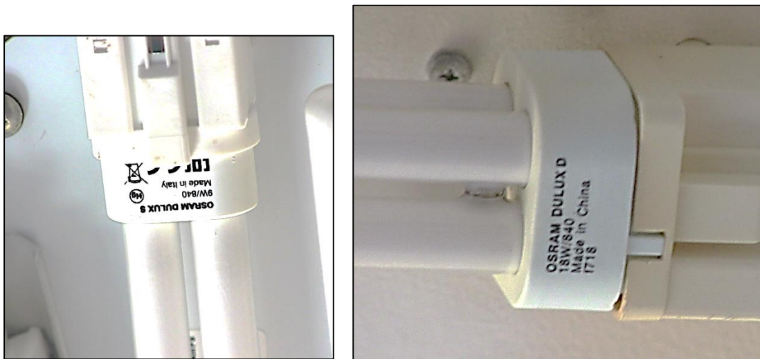
Figure 4.3: CFL bulbs fitted in the student rooms (Lokailwe, 2019)
