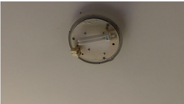
Figure 4.5: Lamp fitting mounted on the ceiling
