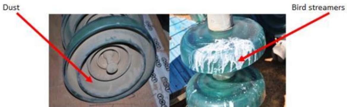
Figure 2.14: Examples of surface contamination of glass insulators
