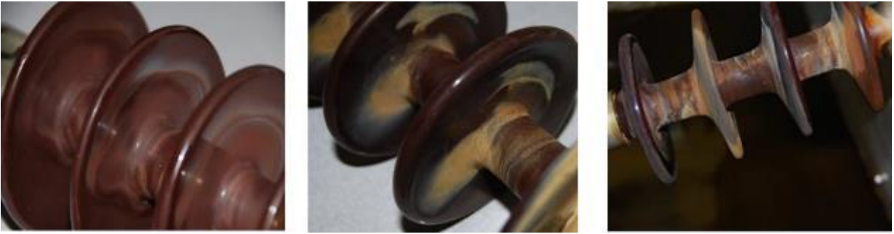
Figure 2.6: Comparison of material aging of a porcelain insulator under HVAC, positive HVDC and negative HVDC excitation, respectively (From Limbo, 2009)
