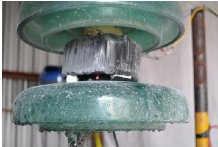
Figure 5.10: Leakage current test setup showing the pollution on the outside of the LCPR1 sensor and insulators (with two stand-off insulators) after testing
