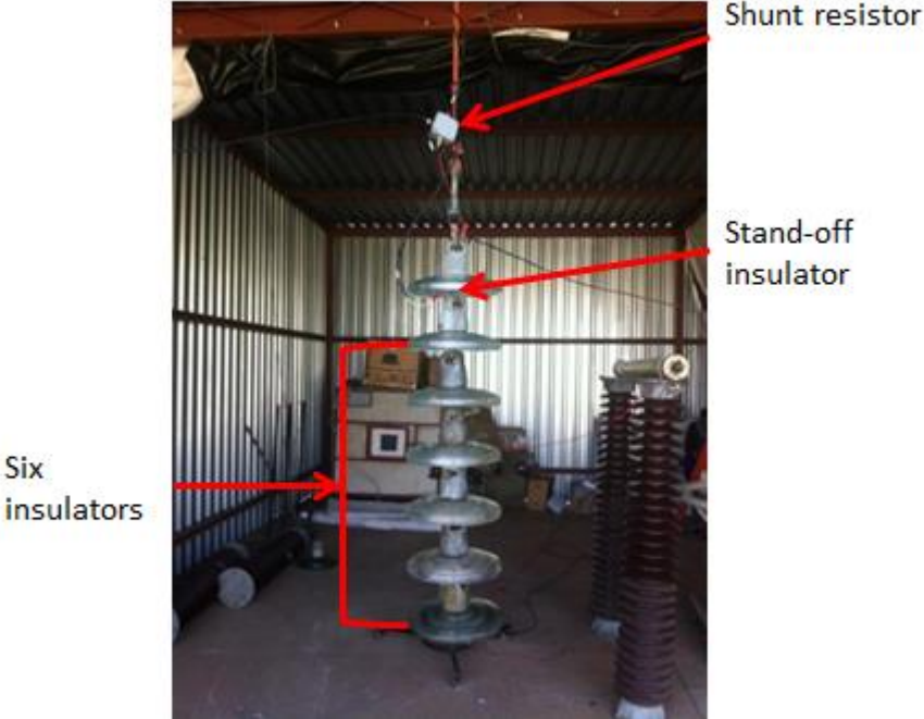
Figure 5.15: Six glass insulators in a string (including the stand-off insulator)
