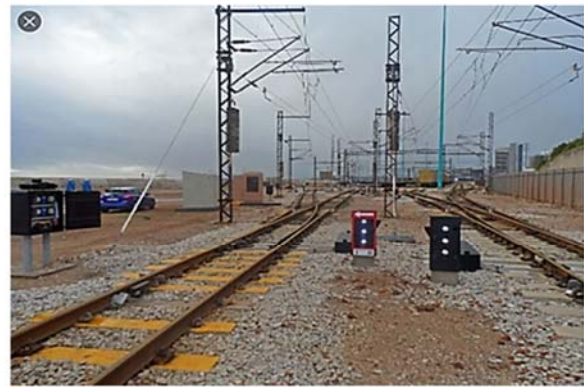
Figure 2-1 (b): Yard control equipment installed at Foreshore, Port Elizabeth
