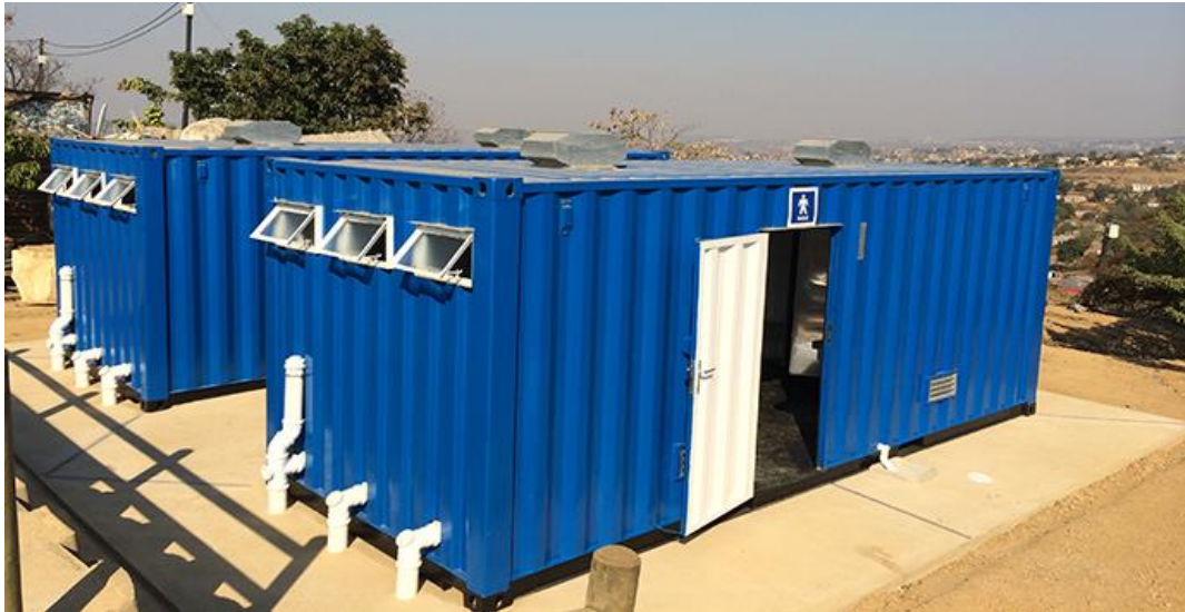
Figure E.4: Communal Ablution Blocks (CABs)
