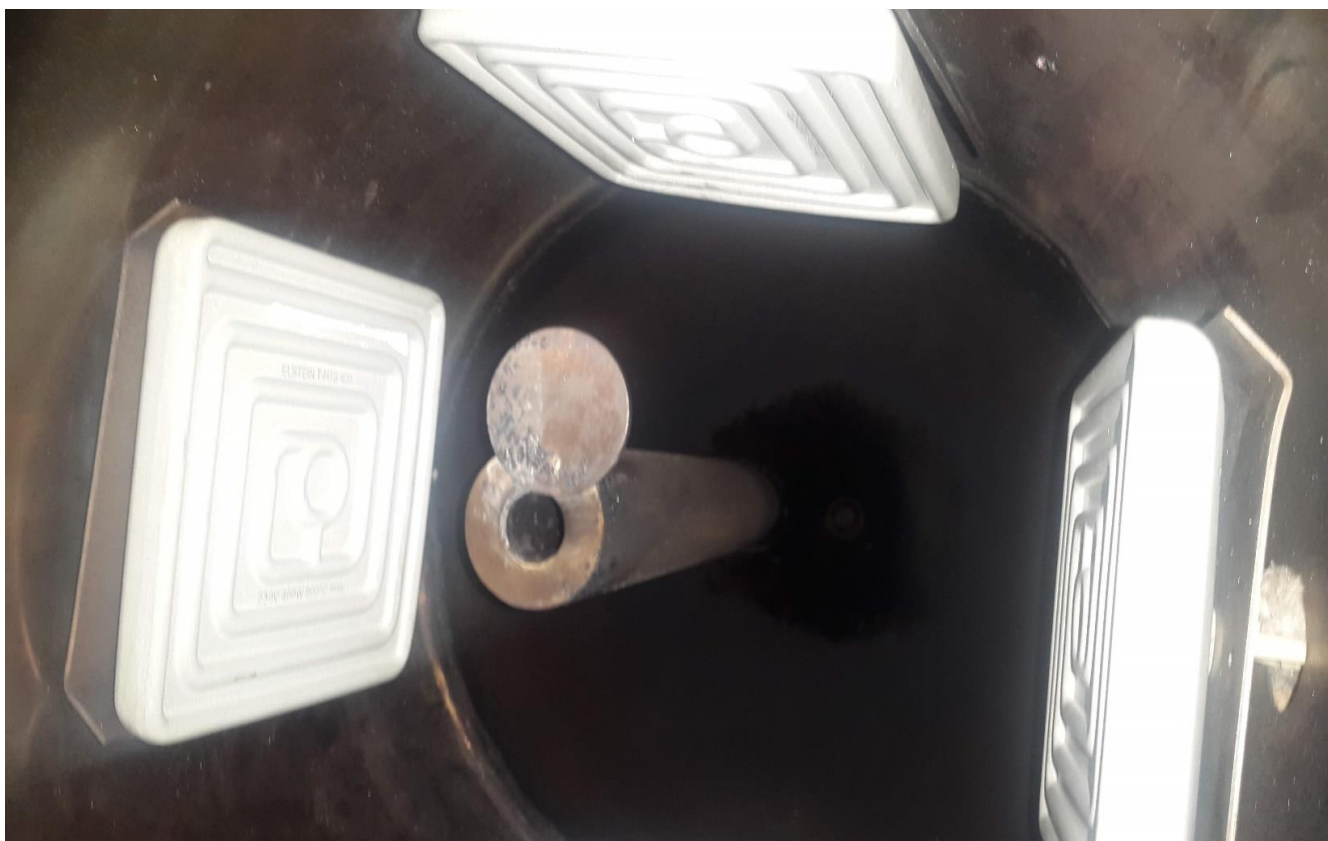
Figure 8-8: Ceramic Heaters Mounted on the reactor
