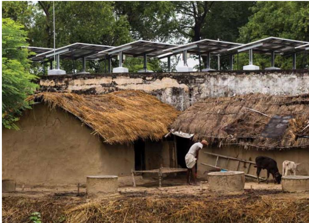
Figure 6. 1: Solar microgrid installation, Dharnai - India (Greenpeace, 2014)
