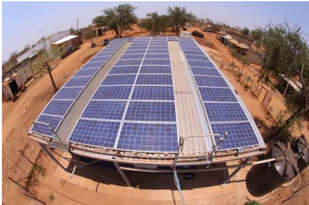
Figure 6. 2: Microgrid (13.5 kW) in Makueni County, Kenya (UoSouthampton, 2013)
