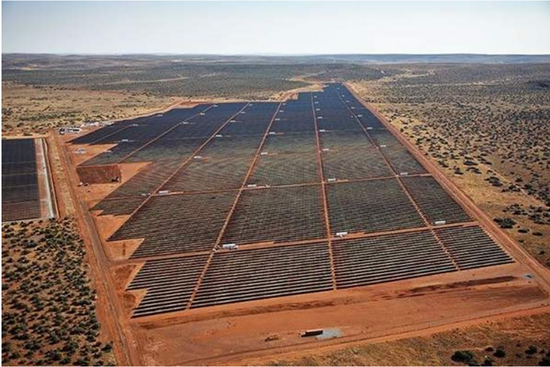
Figure 2.12: The Jasper solar power plant in the Northern Cape, South Africa (From Renewable-technology, 2016)
