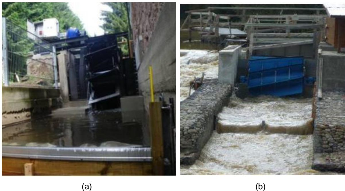
Figure 3.20: Two installations of the hydrostatic pressure machine (HPM): (a) in Bavaria (Linton, 2013). (b) in Bulgaria (Licari et al., 2020)
