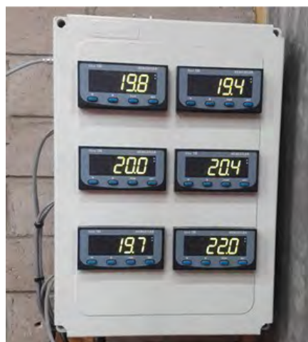
Figure 3.3-2: Battery room temperature monitoring
