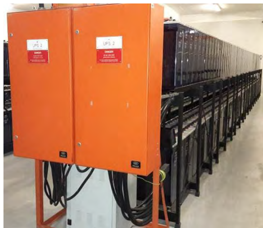
Figure 6.5.3-2: Current fused LA-BESS transition box
