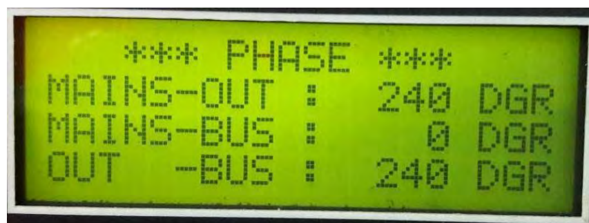
Figure 2.10.2: Four-line LCD - Mains OUT and BUS synchronization
