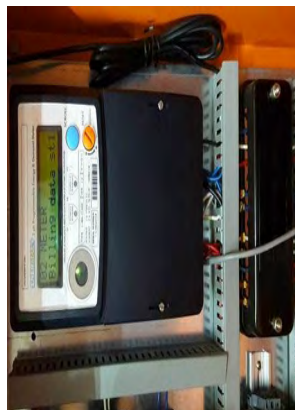
Figure 3.1.3: Enermax energy meter
