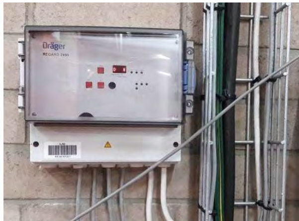
Figure 3.3.3-1: Dräger Regard-2400 controller
