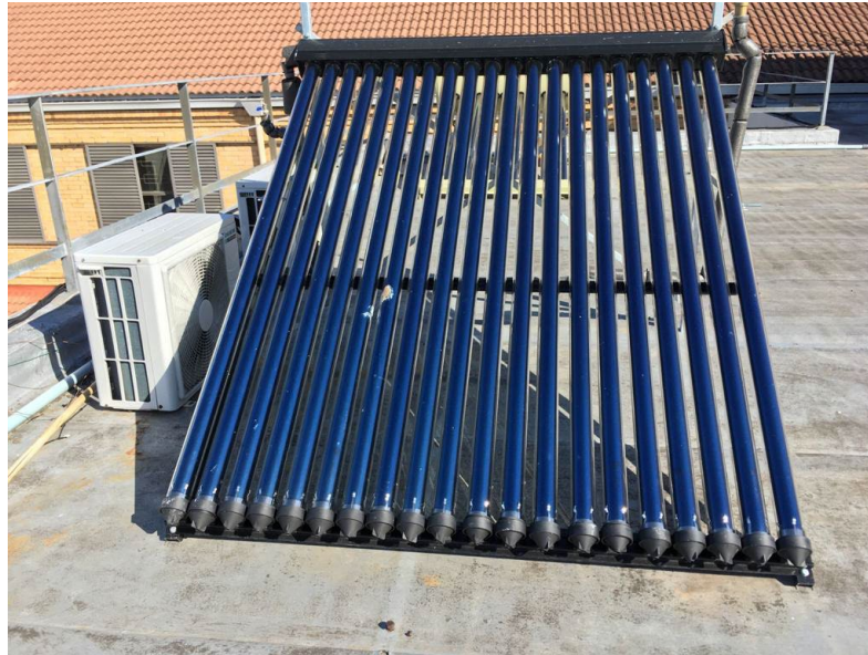
FIGURE 3.9: INSTALLED ETC UNIT
