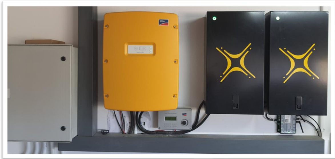
Figure 30: Malmesbury Smallholding - 8kW battery inverter, 2x 3.7kWh lithium batteries and distribution board
