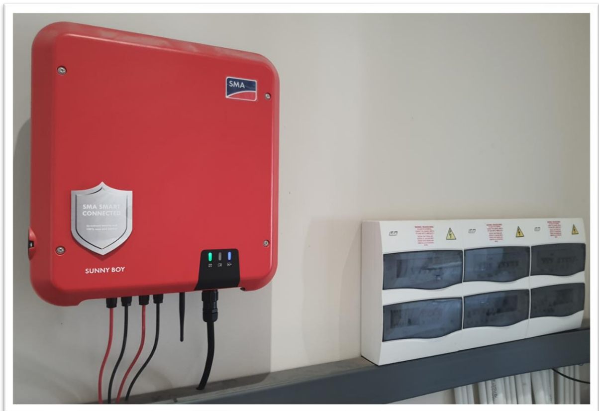
Figure 29: Malmesbury Smallholding - 5kWp PV inverter
