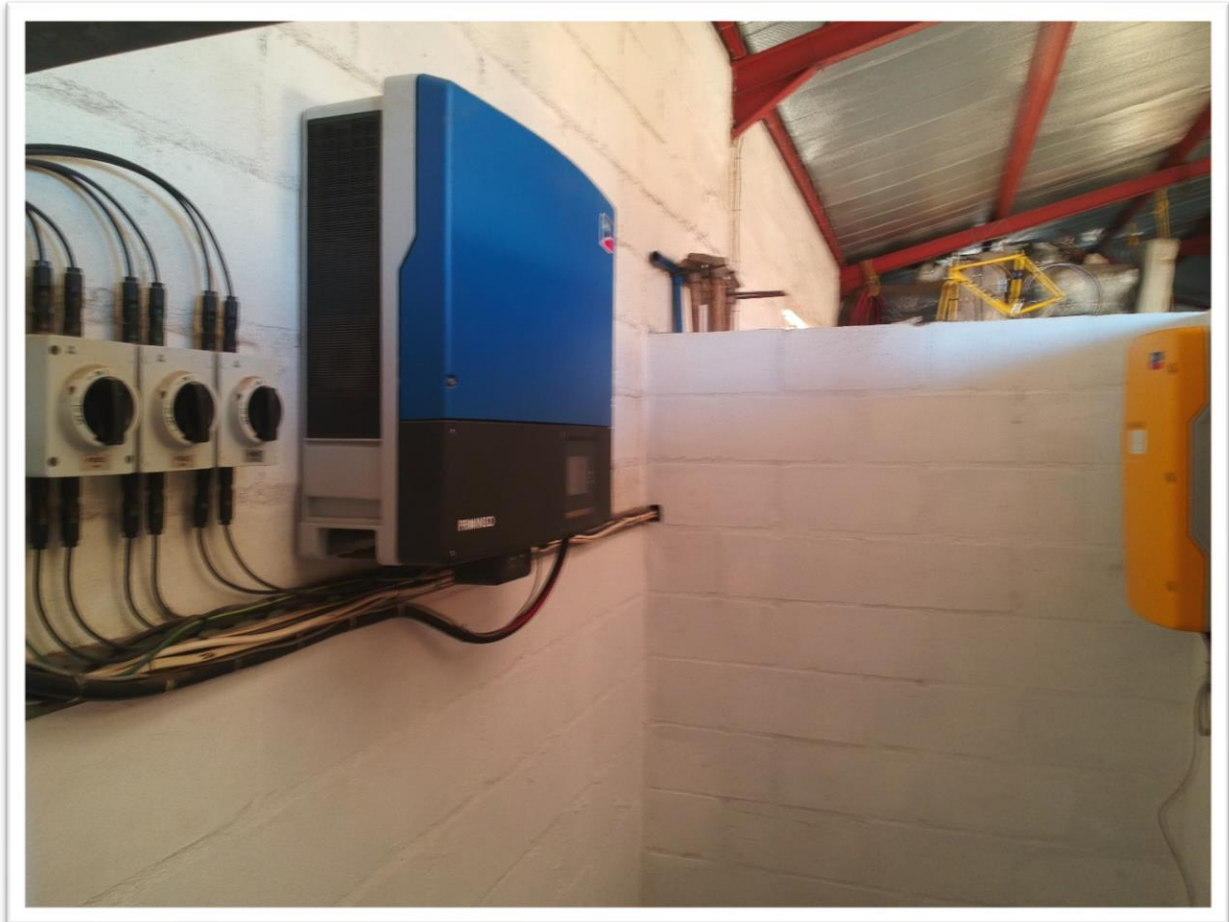
Figure 6: Malmesbury farm SMA Sunny Tri Power 15000TL-30
