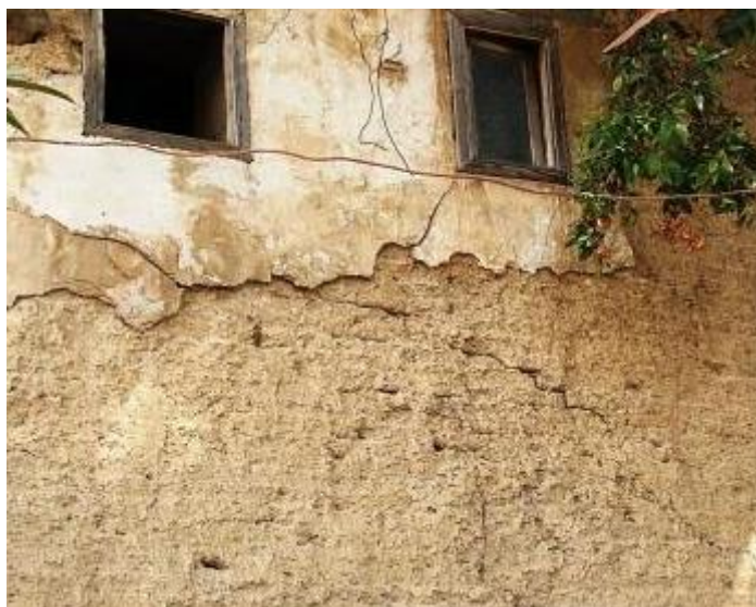
Figure 2.2: Cracking of a structure in Cyprus built with adobe bricks (Illampas et al., 2017)
