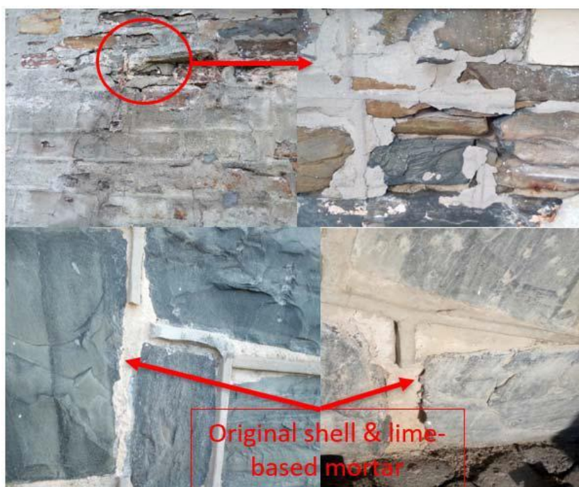
Figure 2.3: Repairs done with incompatible material at Robben Island, causing further damage (Loke et al., 2019)
