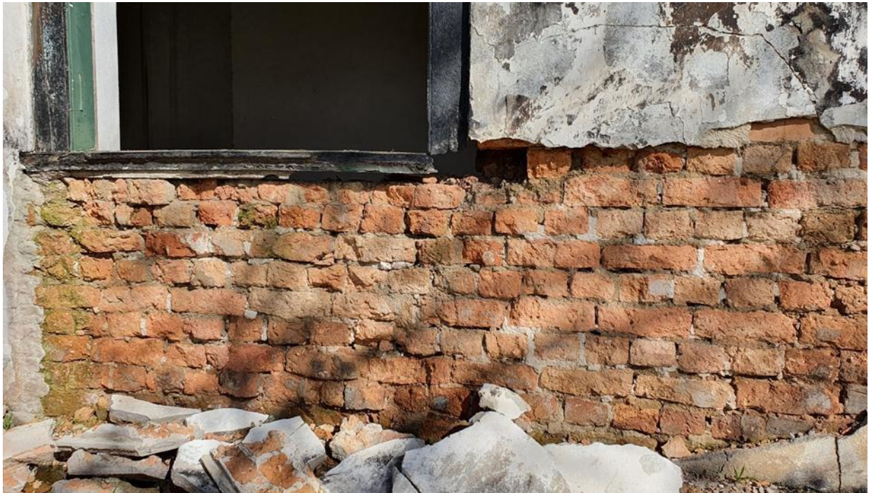
Figure 3.16: Plasterwork breakout on east wall panel exposing the masonry bricks
