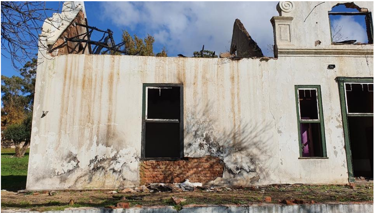
Figure 3.14: Visual damage on the eastern section of the gable wall
