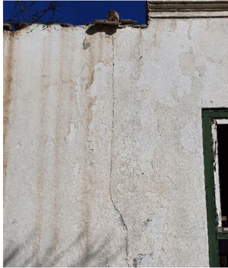
Figure 3.15: Cracking between east and centre wall panels
