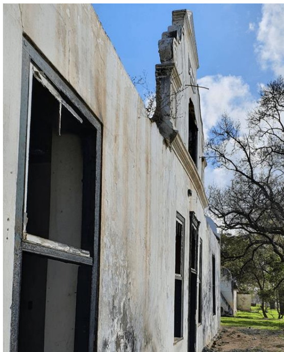
Figure 6.10: Out-of-plane deflection above the architectural ridge of the gable wall
