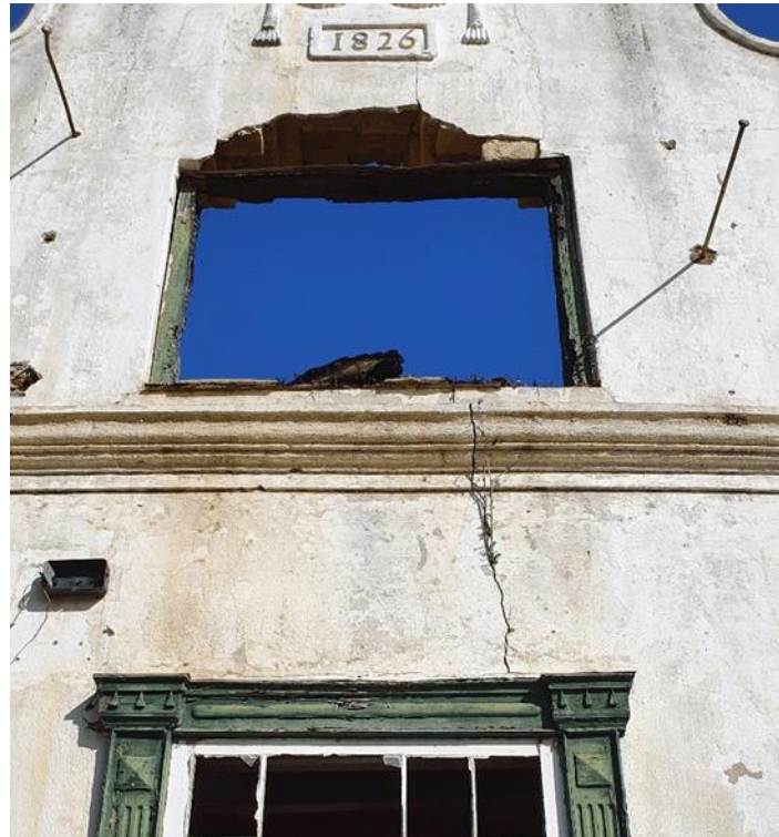
Figure 3.17: Gable crack indicating separation
