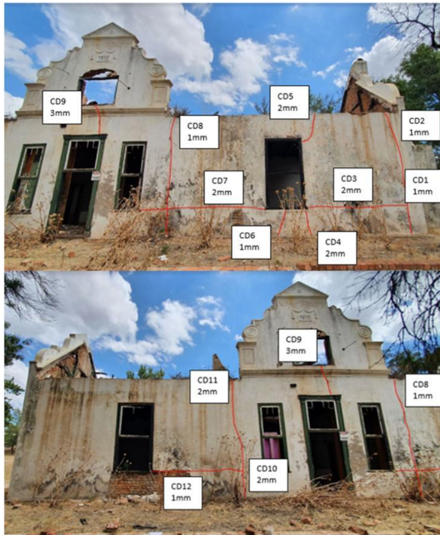
Figure 6.6: Crack depth measurement positions and corresponding crack widths
