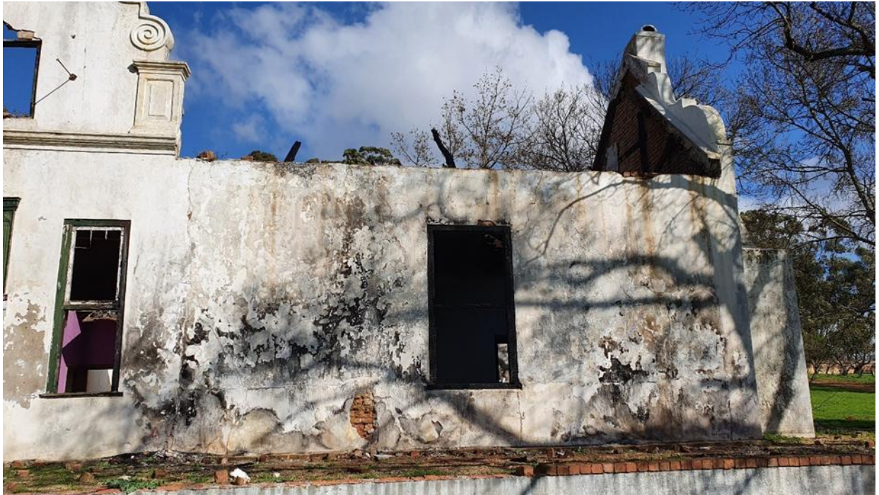
Figure 3.18: Visual damage on the western section of the gable wall
