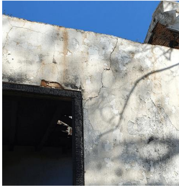
Figure 3.19: Diagonal crack above window of the west wall panel
