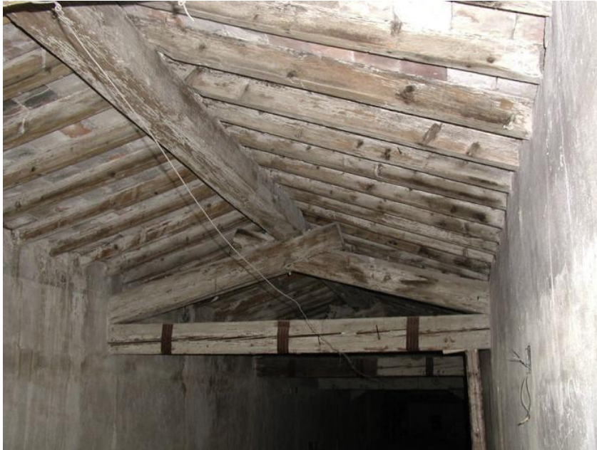
Figure 2.1: Substandard fastening of a truss tie (Tampone and Ruggieri, 2016)
