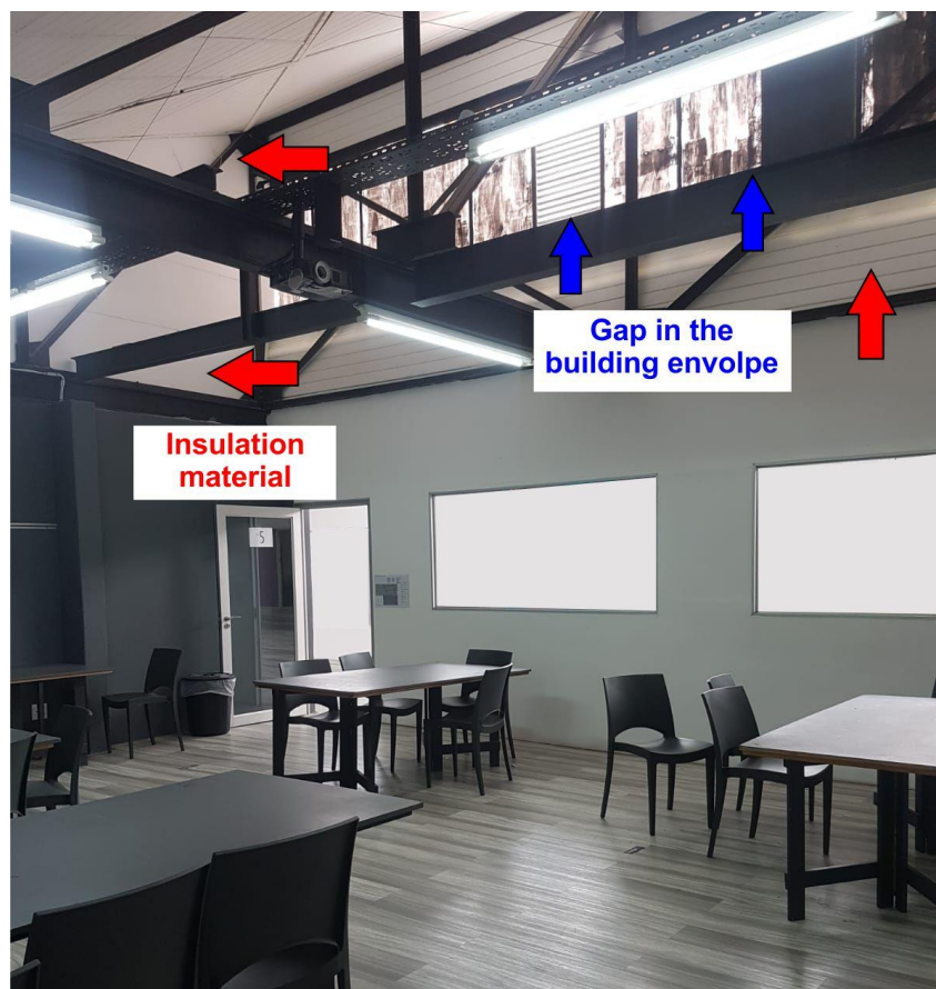
Figure 33. Sound proofing material.
