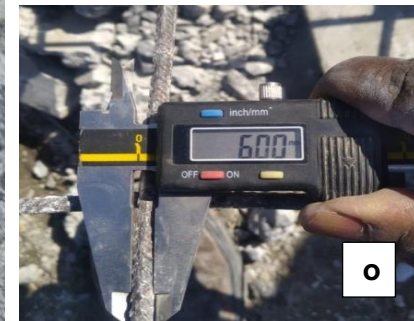
Steel observation after destroying the panel with hammer.
