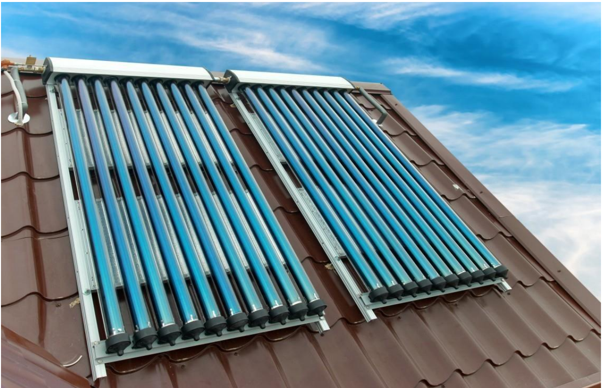
Figure 3.3.1.2.1: A solar thermal panel mounted on a roof. [50]
