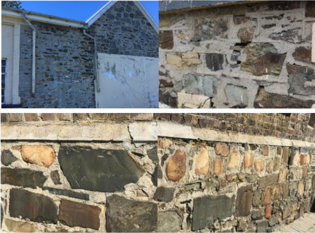
Figure 1.2 Faulty mortar repairs on some buildings on Robben Island
