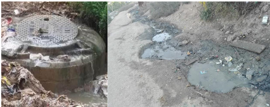
Figure 1. 1 : Sewer Overflow (Picture Taken in Enkanini Informal Settlement, in Stellenbosch)
