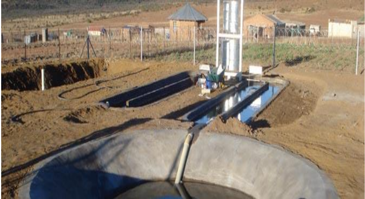
Figure 2.4: Installed biodigester system in the Upper Thukela Area and Richmond area of Kwa-Zulu Natal (Source: SACN, 2009)
