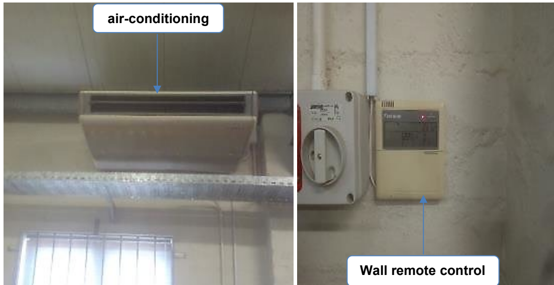
Figure 3-24: air-conditioning inside of laboratory.
