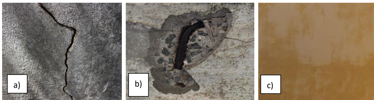
Figure 4.1 Image dataset sample of (a) crack, (b) spalling and (c) intact areas.
