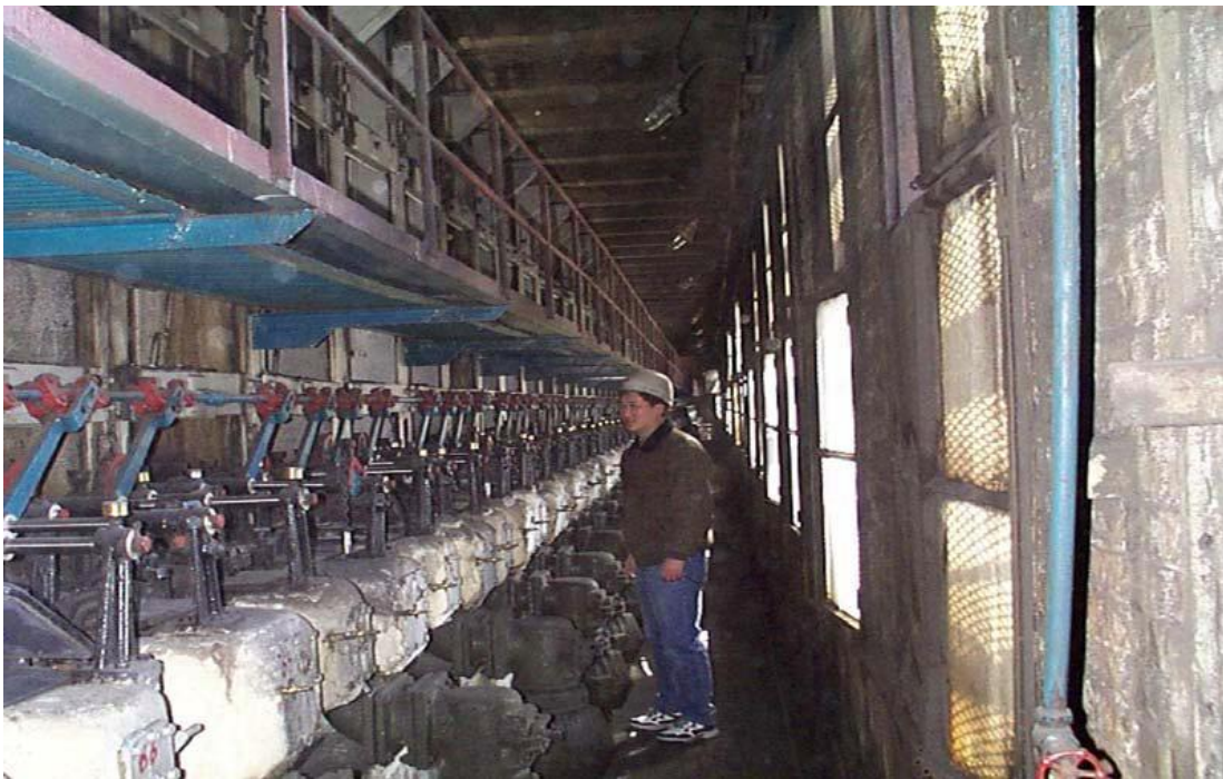
Figure 1.7 Coke oven bottom work environment
