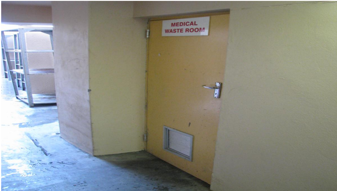
Figure 4.12: Pharmaceutical waste storeroom without proper signage
