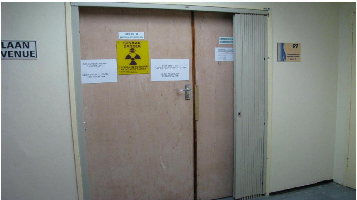
Figure 4.9: Radioactive waste storeroom without proper signage
