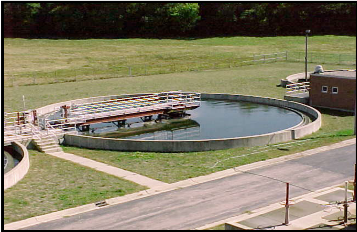
Figure 2.4: Secondary settling tank (MPWWTP, 2012)
