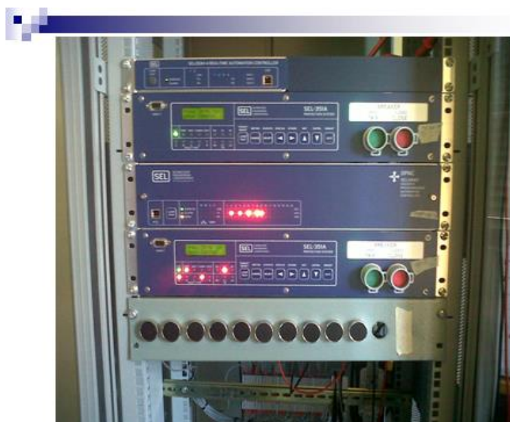
Figure 4.8: Picture of the IEC 61850-based DA system test system panel
