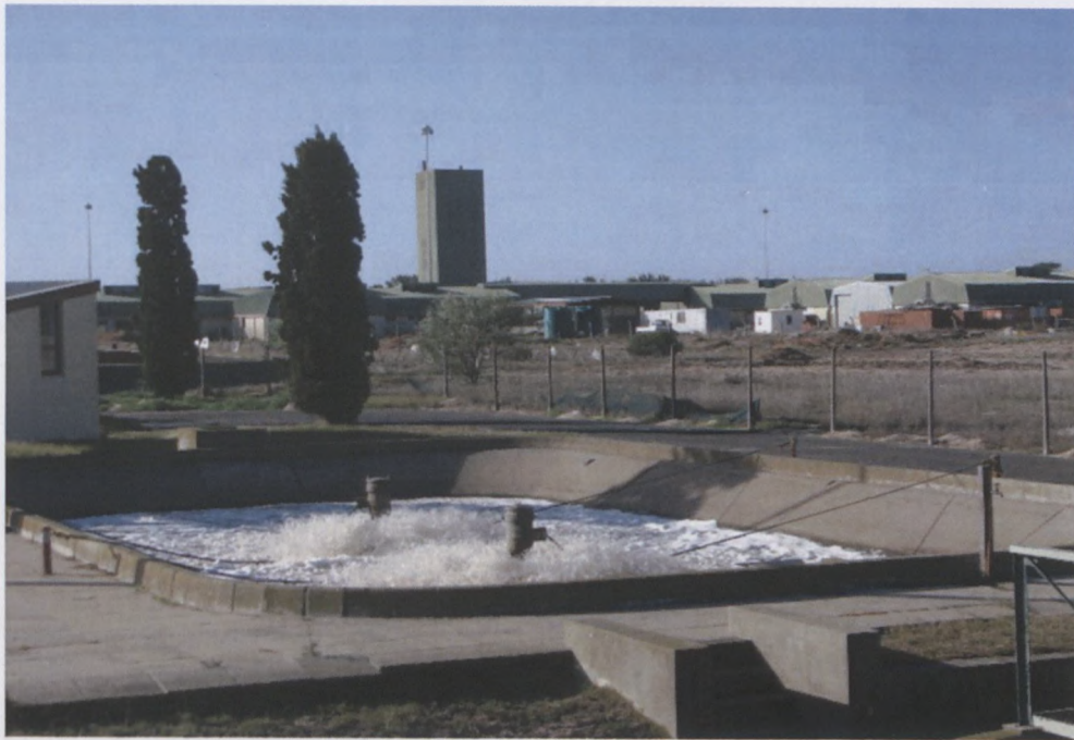
Figure 4.42: MRC Sewage Treatment Works (STWs)
