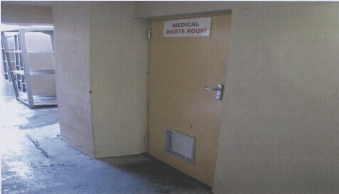
Figure 4.12: Pharmaceutical waste storeroom without proper signage
