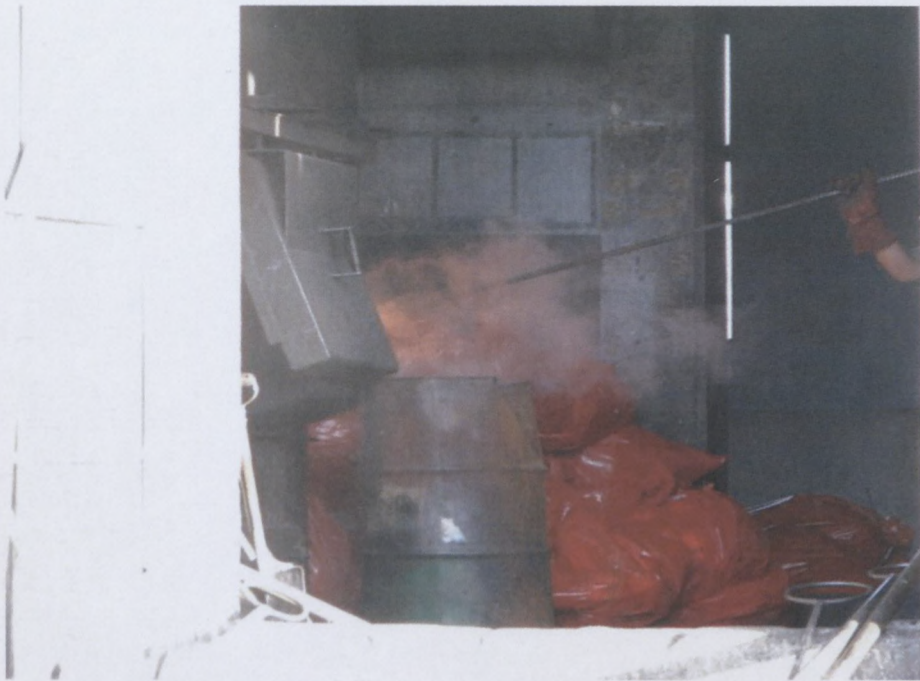
Figure 4.34: Hot bottom ash removed manually and escaping to the atmosphere
