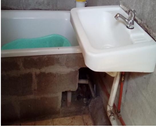
Fig. 8 Represent shoddy works, baths left without trap door for water overflow.
