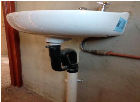
Fig. 21 Represent a complete basin with an S-trap pipe underneath and a flexi, water pipe and a tap.
