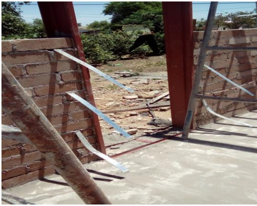
Fig. 12 Represent typical hoop-irons positioned correctly every fourth course and the typical external door frame positioning.
