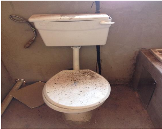
Fig. 20 Represent a typical complete toilet set installed correctly along is the baths trap installed.
