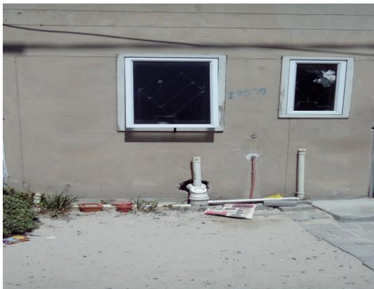
Fig. 3 Represent damaged defective sewer pipe and opened wall.
