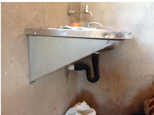
Fig. 19 Represent the zinc supported by bracket on either sides, tap and P-trap pipe underneath.
