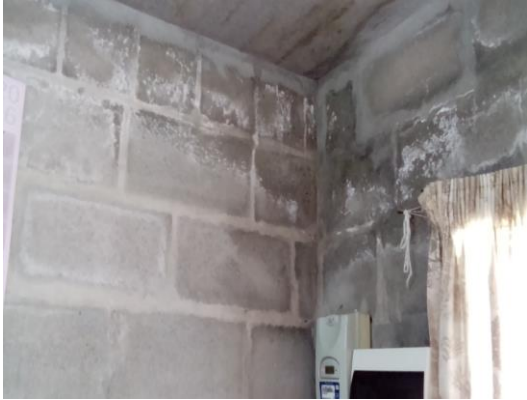
Fig. 5 Represent humid walls through moisture.
