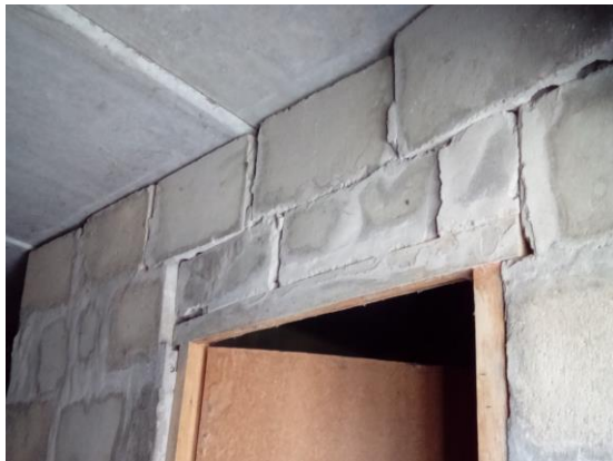
Fig. 6 Represent structural wall defects due to poor resultant quality.
