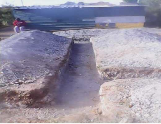
Fig. 1 Represent excavation of 400mm x 600mm footing of a 40m 2 meter BNG house.
