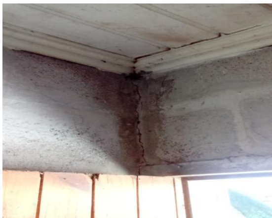
Fig. 7 Represent structural wall defects due to poor resultant quality.
