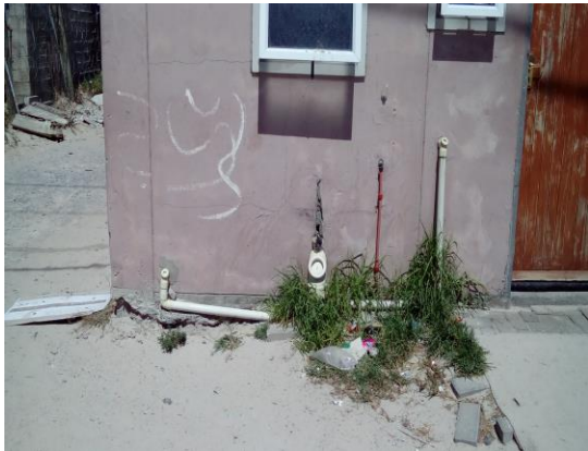
Fig. 2 Represent damaged sewer pipe.
