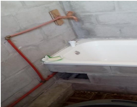
Fig. 10 Represent a typical water connection of the bath tap and the position the tap is being installed.
