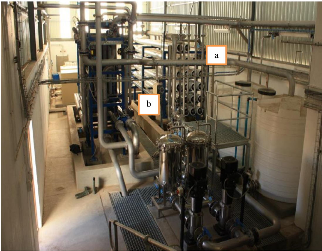
Figure 3.2: Membrane system at the Beaufort west WWTP. (a) Reverse osmosis, and (b) ultrafiltration (Ivarsson & Olander, 2011)
