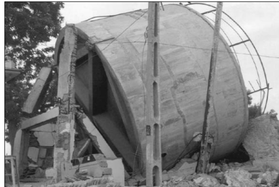
Figure 1.2: Damaged support to elevated concrete water reservoir, 2001 Bruj (Adapted from NZSEE, 2009)
