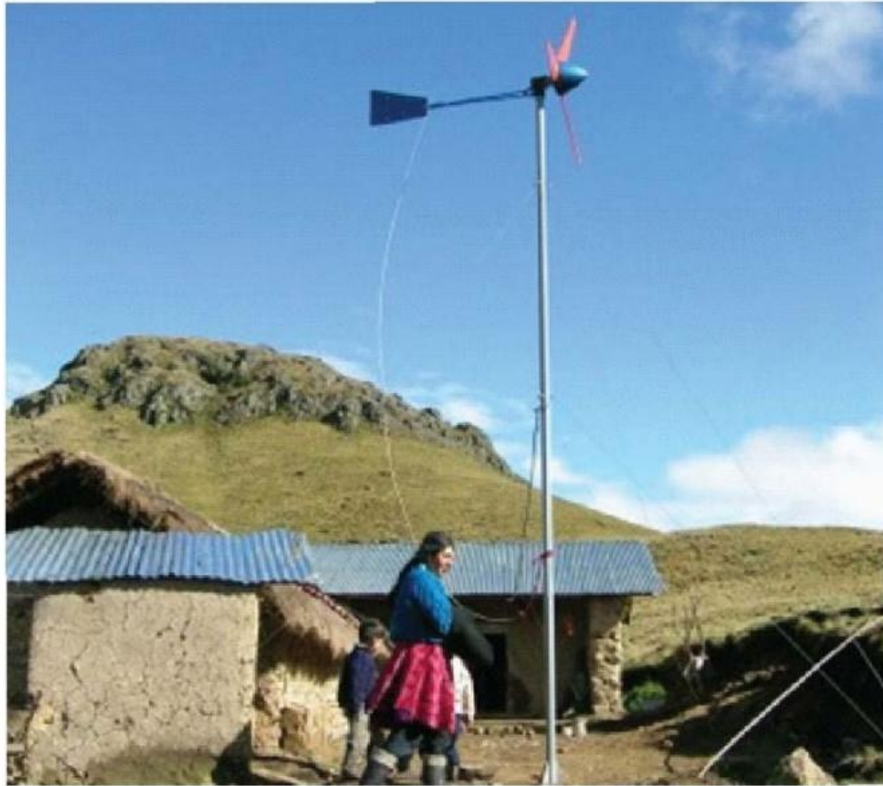
Figure 2.7: A small wind turbine installed in El Alumbre, Peru, set against the backdrop of the Andean Mountain range rising to approximately 4000 meters (Soluciones Practicas, 2013)
