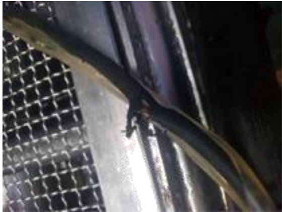
Appendix 4.3. A cable damaged in rough terrain
