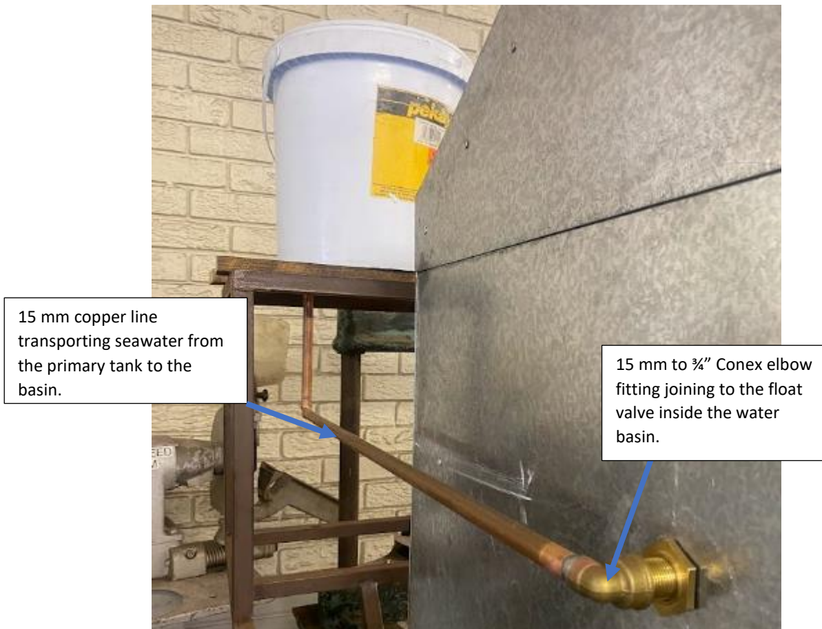
Figure 3.18: Saline water tank to basin connection
