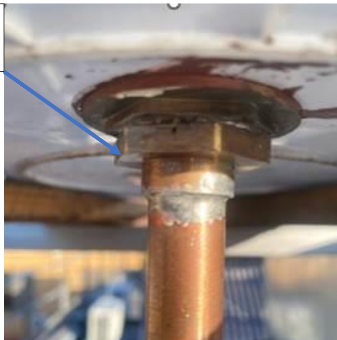
Figure 3.10: Primary tank outlet
