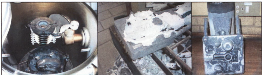
a. Damaged Coil
