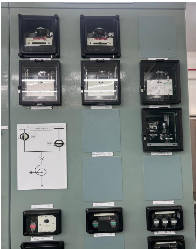
Figure 1.1: Currently Installed Protection
