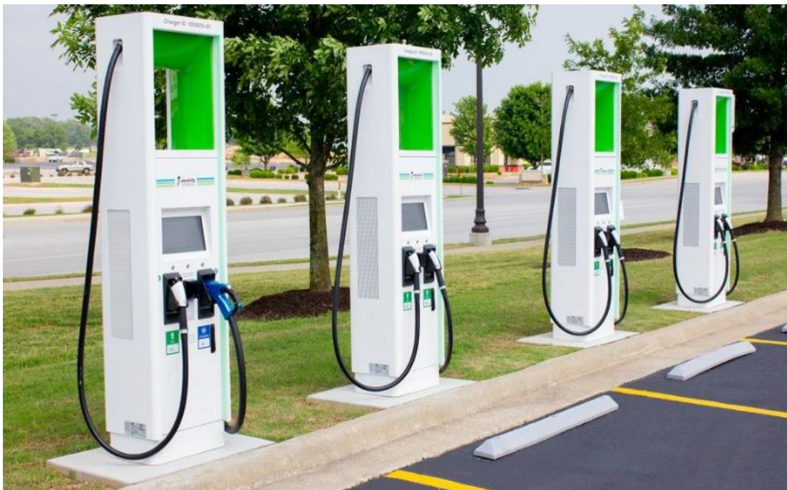
Figure 2.3: EV DC Charger stations.
