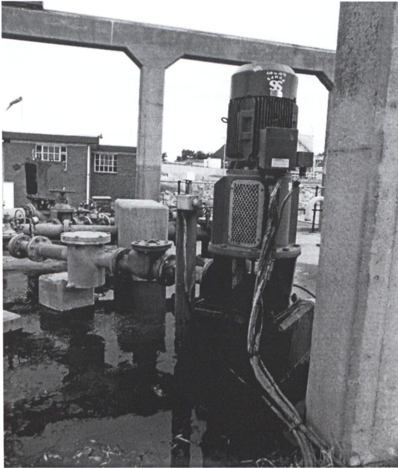
Fig. 3.10 Multistage centrifugal pump and its leakages
