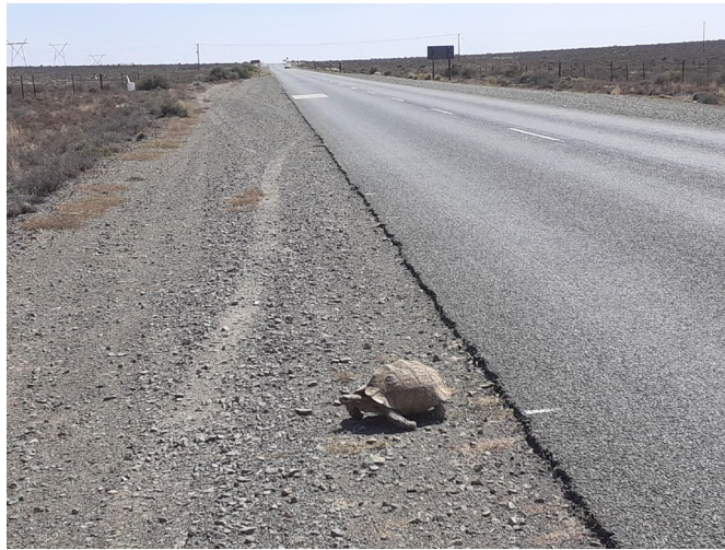
Figure 6: Shoulder drop more than 50mm (Western Cape Government photos, 2021)
