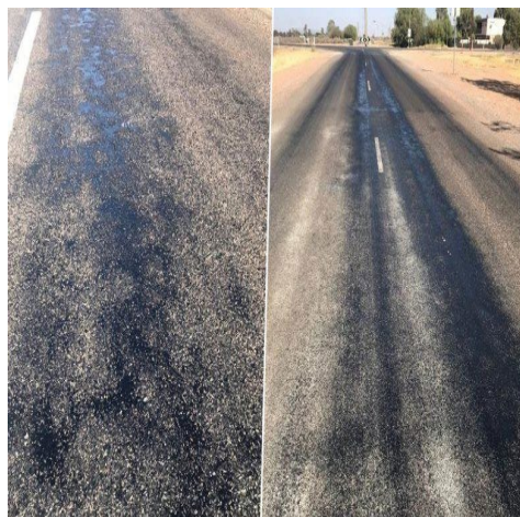
Figure 12: Aggregate loss resulting to bleeding TR33/5 (Western Cape Government photos, 2021)
