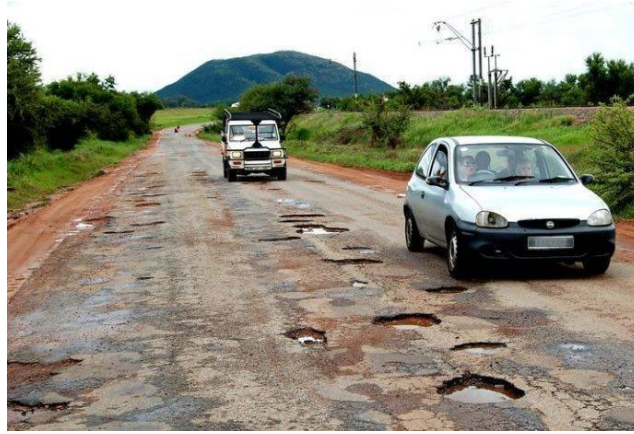
Figure 1: Examples of pavement deterioration (Arrive Alive, 2019).
