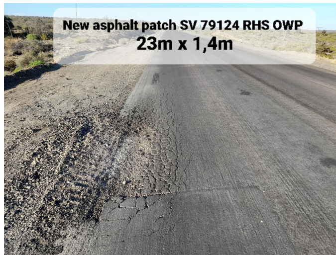
Figure 8: TR33/5 crocodile cracks with disintegration (Western Cape Government photos, 2021)
