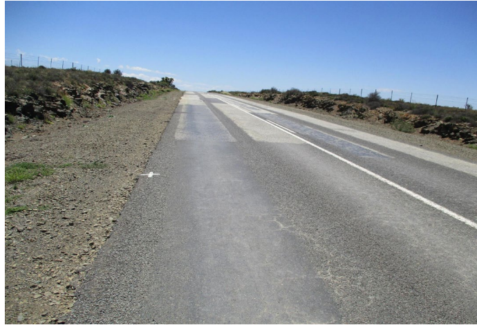
Figure 11: Aggregate loss on the TR33/5 (Western Cape Government photos, 2021)
