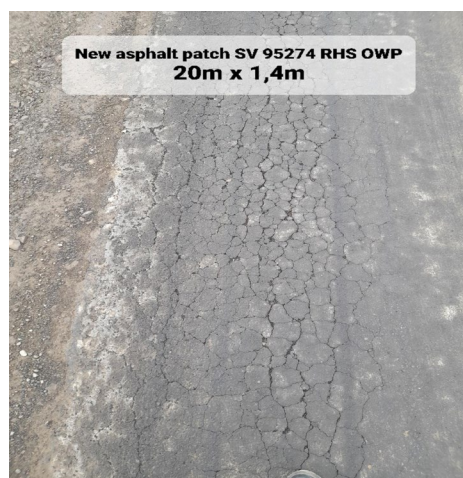
Figure 7: TR33/5 crocodile cracks failure without disintegration (Western Cape Government photos, 2021)
