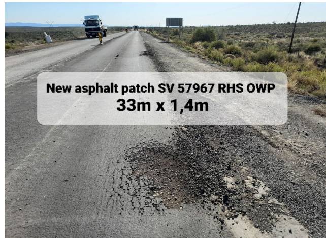
Figure 4: Base failures on the TR33/5 (Western Cape Government photos, 2021)
