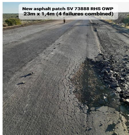
Figure 5: Base failures on the TR33/5 (Western Cape Government photos, 2021)
