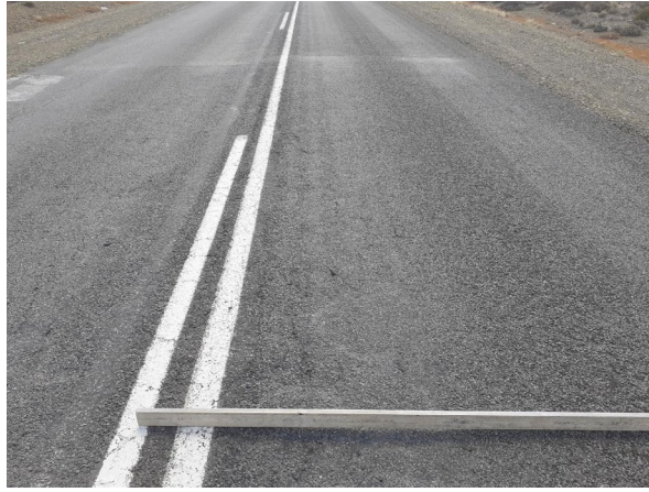
Figure 9: Road rut distress on the TR33/5 road (Western Cape Government photos, 2021)
