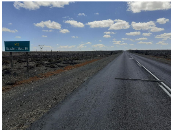
Figure 10: Road rut distress on the TR33/5 road (Western Cape Government photos, 2021)
